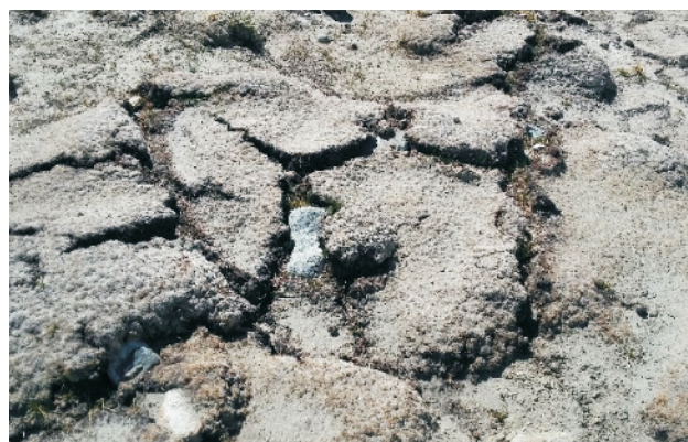
A degraded form of frost heaves showing desiccated conditions
