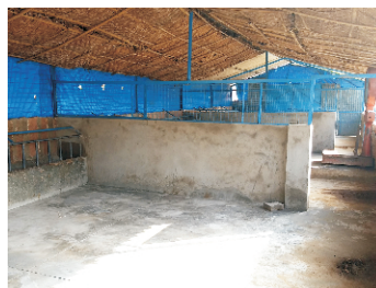
East-west orientation long axis on south side provides plenty of sunlight inside shelter during winter
